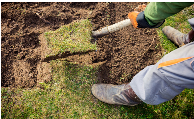
Dig out topsoil a depth of 12.5cm plus the paving slab thickness.
