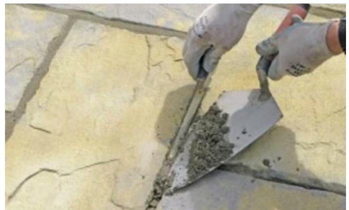
Filling the gaps between the slabs will prevent water and weeds growing between them.
