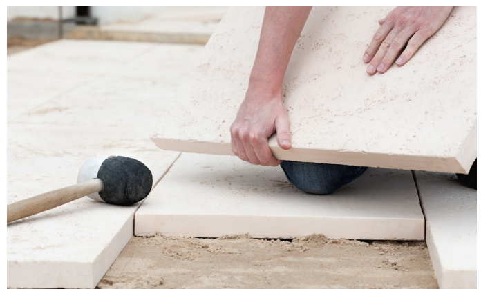
Lay the slabs on dry sand to make sure they fit before fixing them with mortar.
